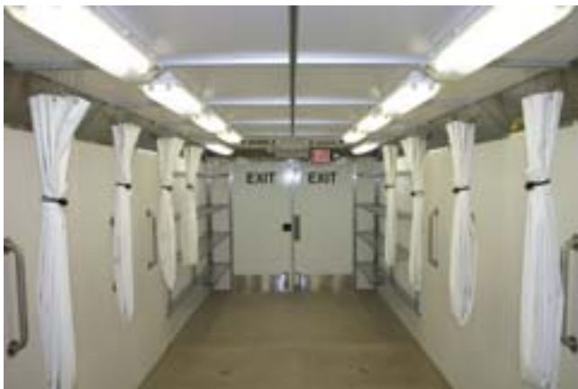
The vehicles' interior shower decontamination area features an automated over/under spray system for ambulatory patients.
